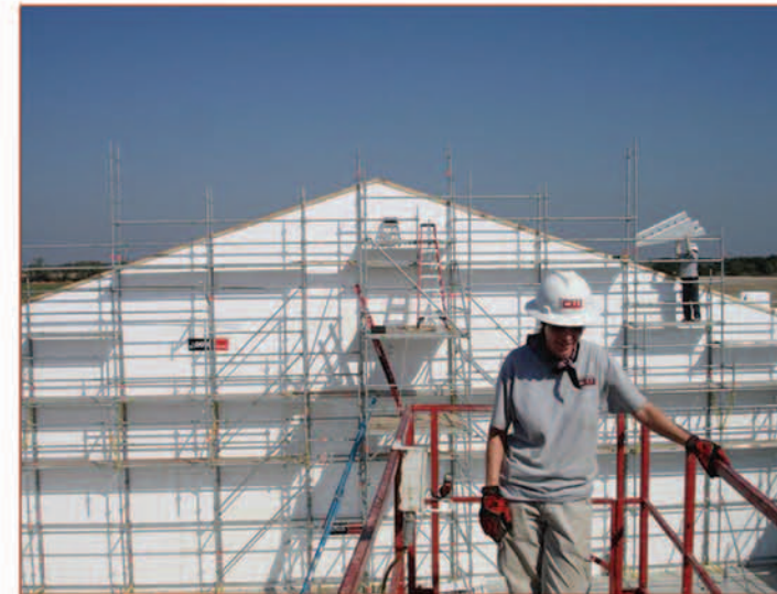
Project Name: New Hope Church, McPherson, KS Size: 2 Story/25,000 square feet ICF Installed: Logix
