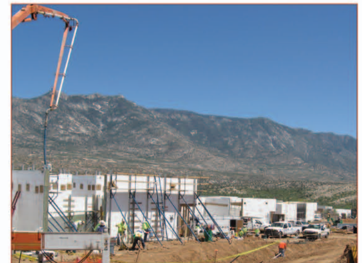
Project Name: Miraval Resort Single Family Development, Catalina, AZ Size: 105,000 gross wall square feet ICF Installed: Amvic
