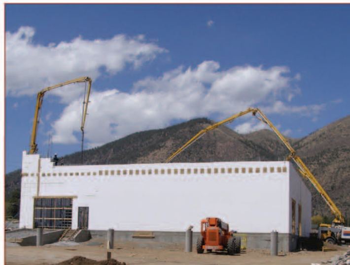
Project Name: Border Construction Supply Office/Warehouse, Flagstaff AZ Size: 12,700 square feet ICF Installed: Amvic
