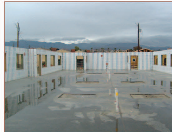
Project Name: Beckett House Assisted Living Center, Lake Havasu, AZ Size: 21,500 gross wall square feet ICF Installed: Arxx
