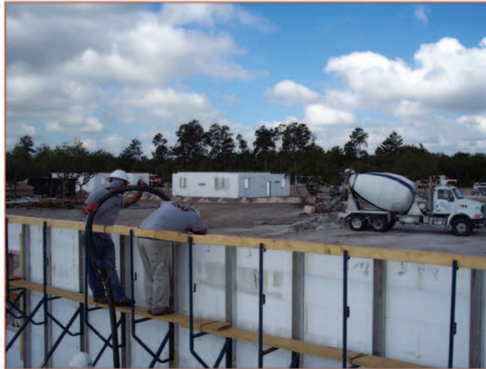
Project : Rafiki Village Corporate Training Center, Orlando FL Size: 13 buildings/25K gross wall square feet ICF Installed: Greenblock
